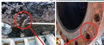
Small groove allowed oil leak
