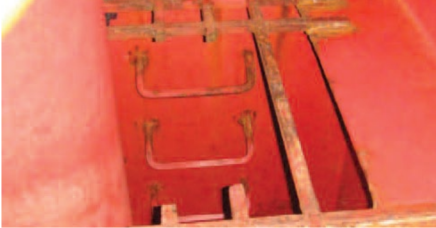
Above: Even a substantial metal grill did not dissuade a number of stowaways who cut through the bars to gain access to this rudder trunk void space
