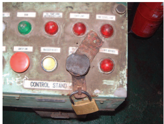
Protective measure to prevent tampering with the luffing limit switch
