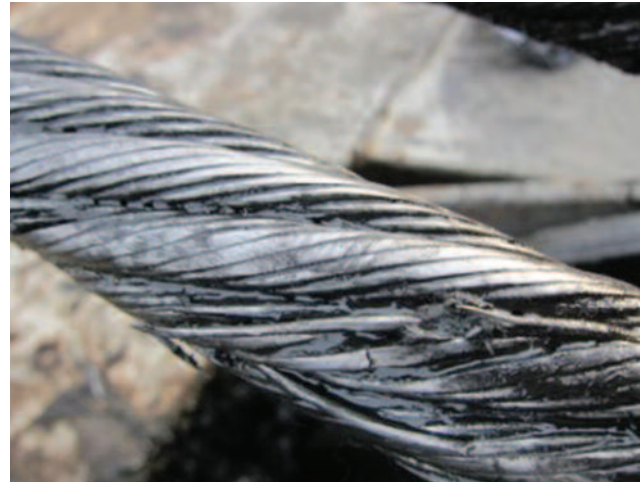
Hoist wire damage
