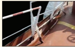
▲ Close up view of damage to sheerstrake and upper deck railings on own vessel
