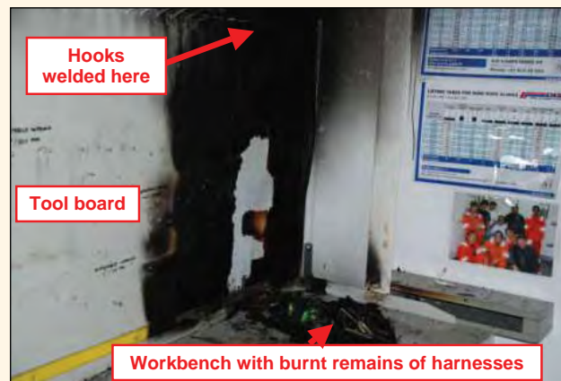
▲ View of interior of deck workshop cum store showing fire damage
