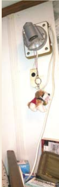
The original light fixture now made operational with new power cord and switch fitting after implementing corrective action
