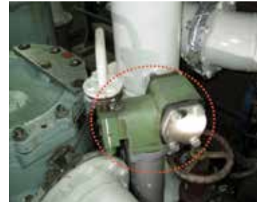
Pressure control valve as installed
