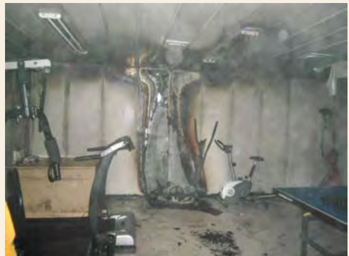
View of fire-damaged bulkhead, deck and deckhead
