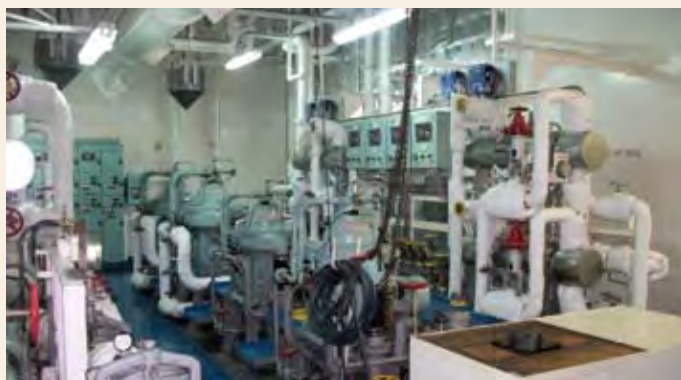
Corrective action #1 implemented – with the purifier overhauling stand positioned correctly
