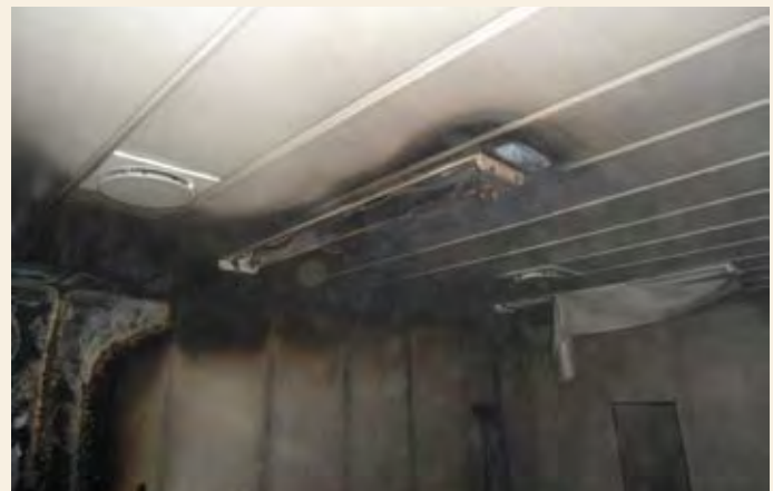
View of damaged deckhead panelling and the light fixture that is thought to have started the fire
