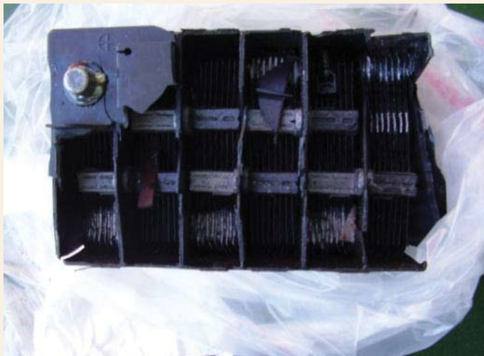
View of battery with shattered top
