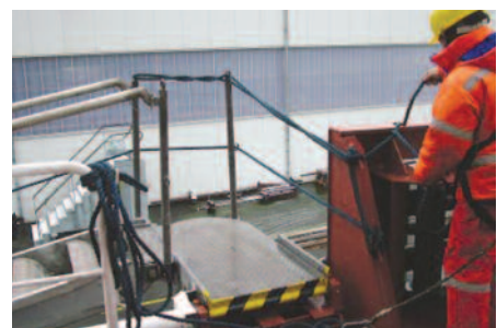
Inadequate guard rail ropes over which a seaman fell to his death (Courtesy MAIB)
