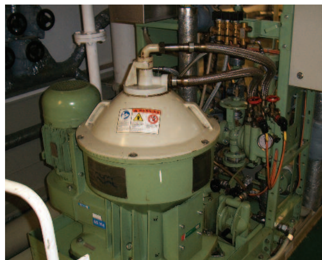
Lubricating oil purifiers extract solid and soluble impurities
