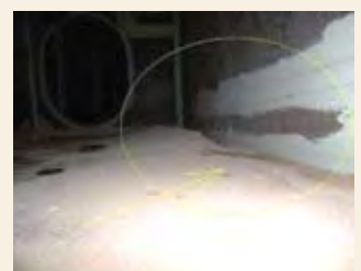
Buckled stringer inside side ballast tank caused by contact in bow region
